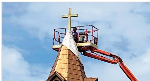
Thanks to the generosity of Capital Campaign donors, repairs were completed on the steeple at St. John the Baptist Church in Morrystown.
